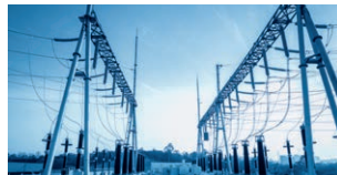
Power transmission and distribution (SF 6 )
