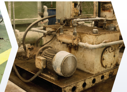
Constantly Running HPU Wastes Energy
