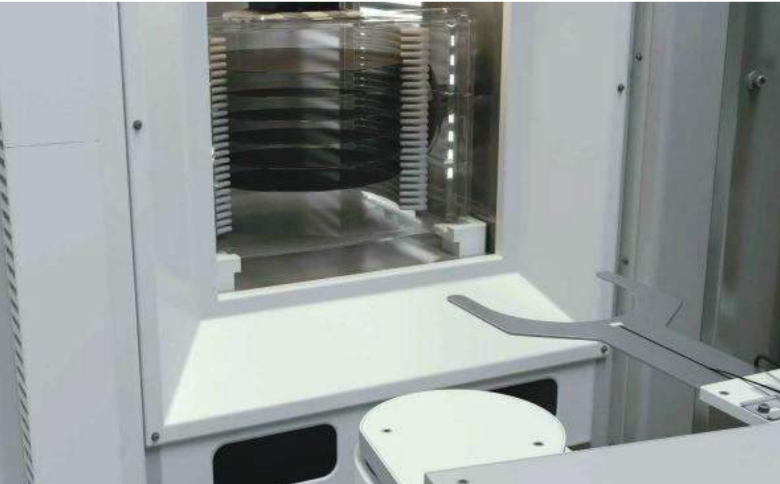
Fiber optic units are used to detect whether wafer is settled on the handler equipment for wafer taping before grinding.
