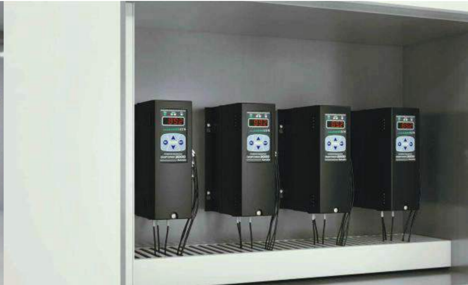
Power controllers are used to control power of heating devices to maintain stable temperature of the cleaning solutions.
