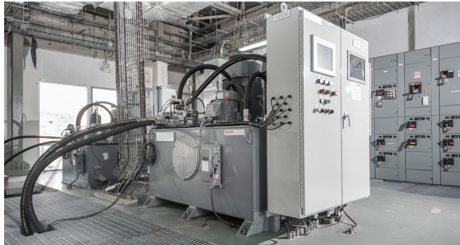
Complexity in applications or specification may require complex control packages nearly the same size as the hydraulic power unit. A well designed and built power unit not only achieves functional criteria but can also be an attractive addition to the production floor.
