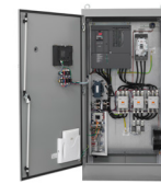
VFD PANELS FOR PUMPS
