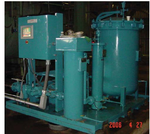
Model KL30 at Power Plant in Oklahoma
